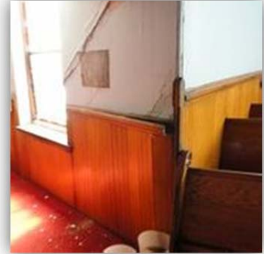
FIGURE 3: SEPARATION OF PLASTER AT CORNERS
