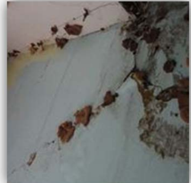
FIGURE 6: FUNGUS GROWING ON WALL
