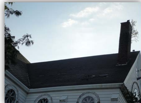
FIGURE 1: TREE GROWING IN CHIMNEY
