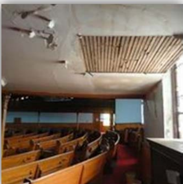
FIGURE 5: WATER DAMAGE TO CEILING
